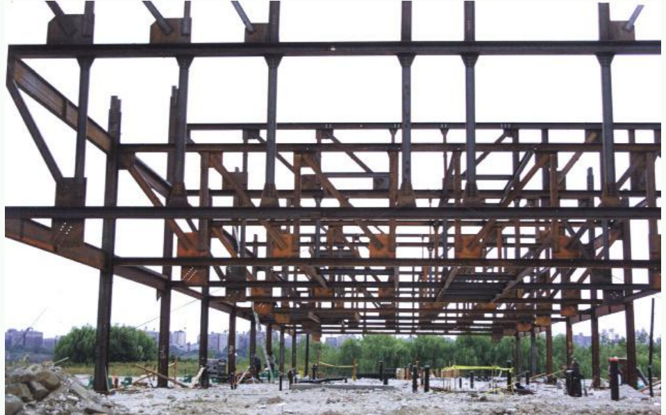
A common ground level view of column-free first floor of staggered truss project.
