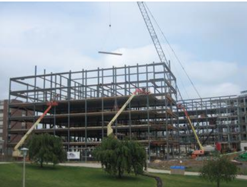
Steel erection at Kutztown University occurred this summer. Lateral bracing is provided by chevron braces strategically located to avoid window locations.
